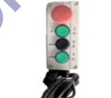
Inspection Box Otis XAA26220AA1/AA6 UP000487
