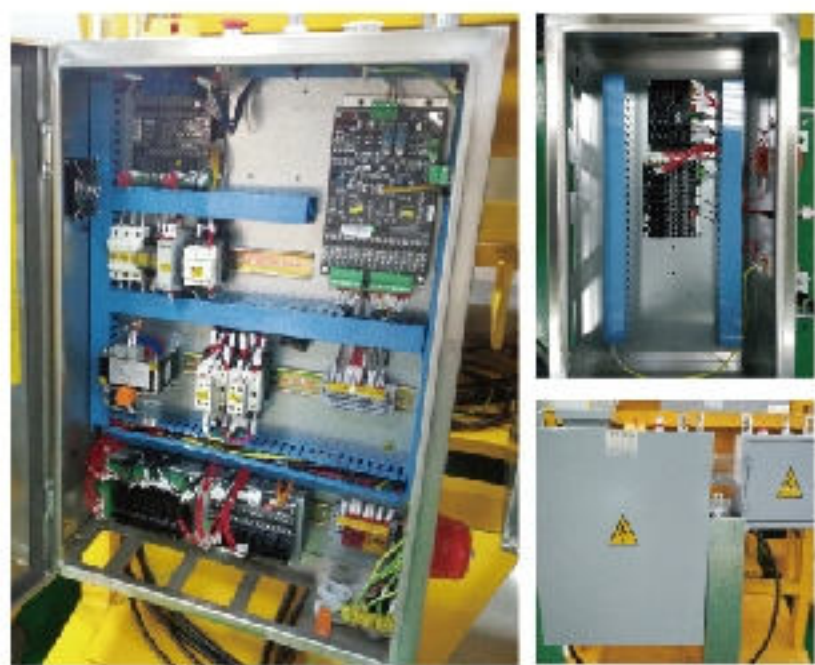
·Escalator control cabinet
